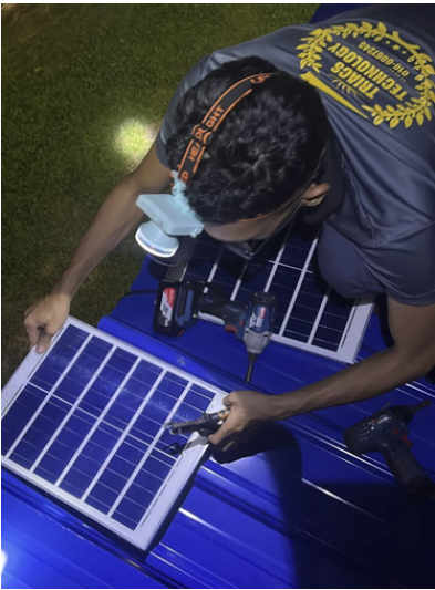
Photo of Solar Panel
